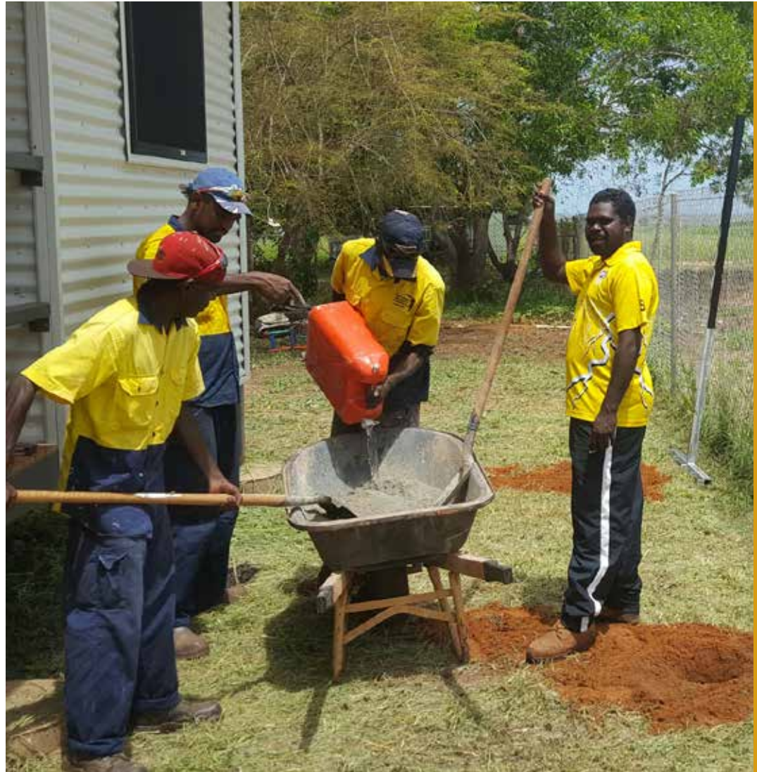
Pictured from L-R Emmanuel Campion, Shaun Morris, Hayden Narragoidj, Cyril Wilson Preparing to concrete in a bush clothesline at Lot 621
